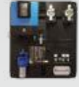
CONTROL STATION PANEL
