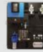
CONTROL STATION PANEL
