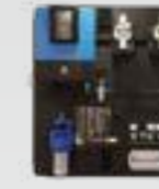
CONTROL STATION PANEL
