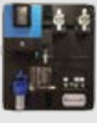
CONTROL STATION PANEL
